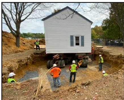
The cottage rolling down a ramp over its new footings in the Park.
