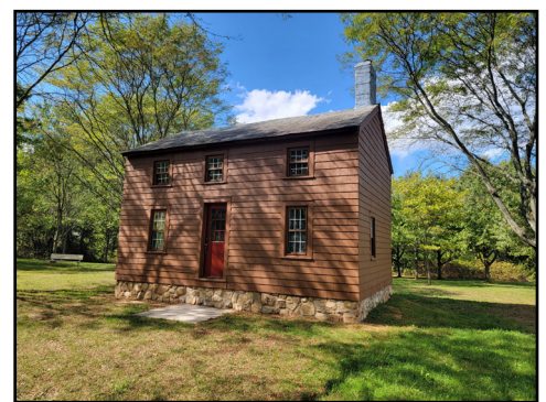
Restoration of the 1713 East Jersey Cottage is ongoing. As of October 2022, the sill plate, stone work, and exterior painting have been completed. The cottage is dark brown with a red door.
